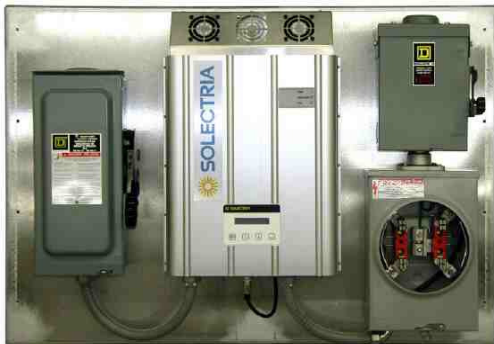
Solectria Inverter on a Prewired Power Panel
